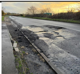
Pothole at the bottom of Essendon Hill
